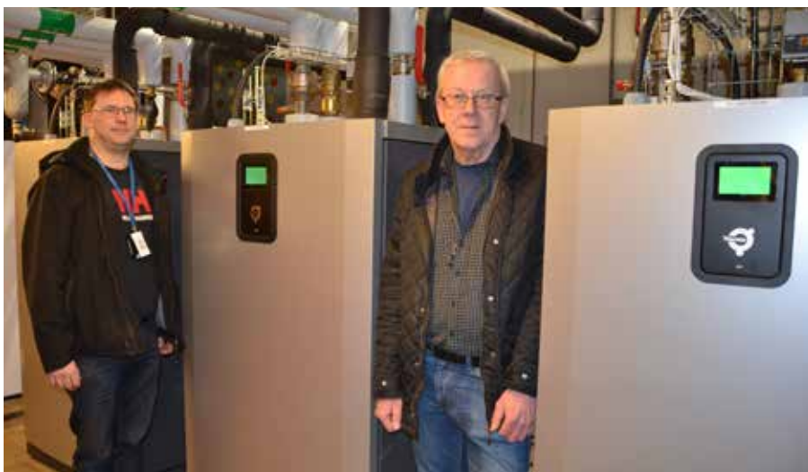
Mattias Berg (left) and Per-Inge Andersson (right) at Thermia Mega heat pumps
