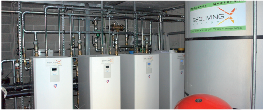
The heating room with Thermia Robust ground source heat pumps
