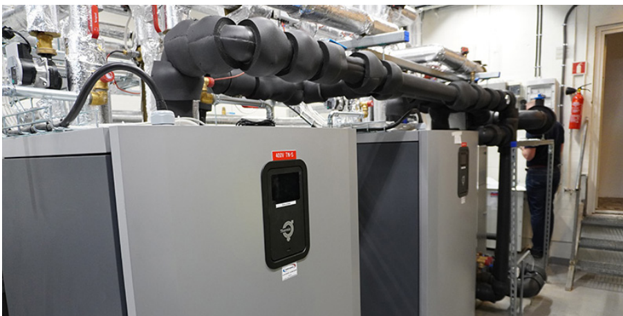
Thermia Mega XL in hotel's machinery room
